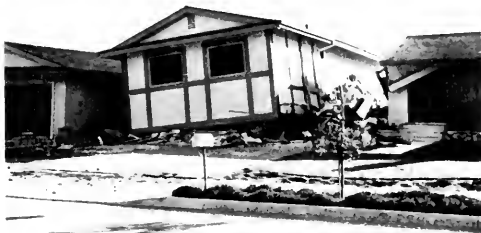
Photo 22. Example of two-story, split-level home where lack of structural support in garage portion allowed collapse. Courtesy of the City of Los Angeles Department of Building and Safety.
